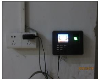
Photo of the inside of the main production hall attendance machine.JPG
