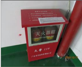
Photo of fire safety equipment fire extinguishers.JPG
