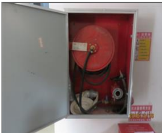
Photo of fire safety equipment fire hydrant.JPG
