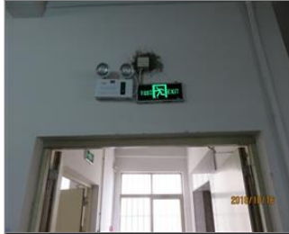
Photo of fire safety equipment emergency exit and emergency light.JPG
